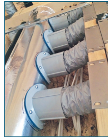
Main trunk and ducts in the wall
