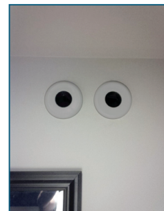
Diffusers on the wall with black collars
